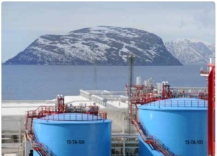
...or storage tanks (Photo: Statoil).
