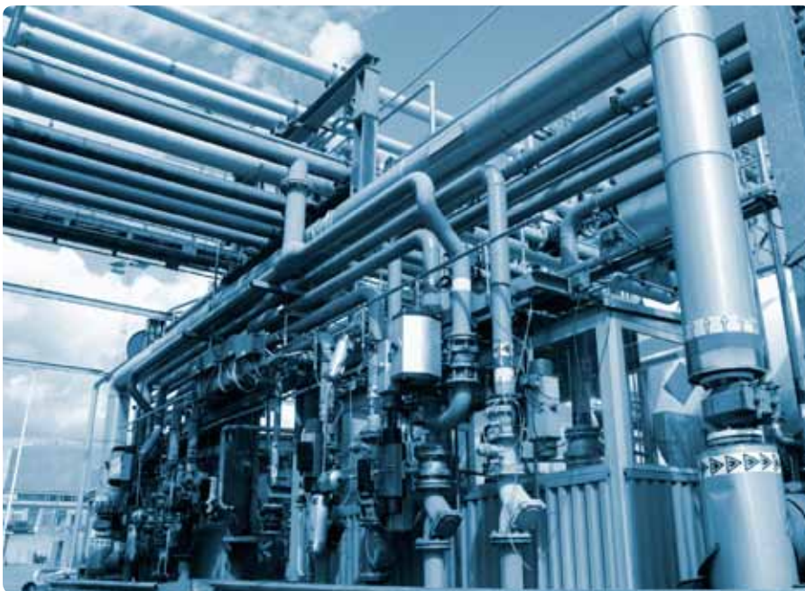
Explosive areas include pipelines...
