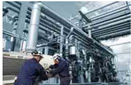
Engineers working on pipelines inside oil refinery
